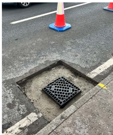
SE NMC: A702 Category 1 repair
