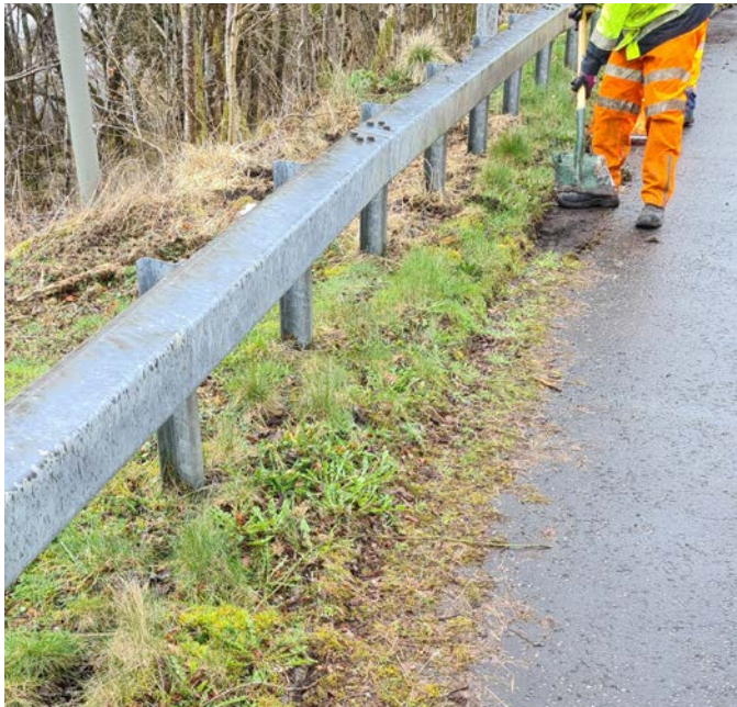
NW NMC: A828 Footway siding out
